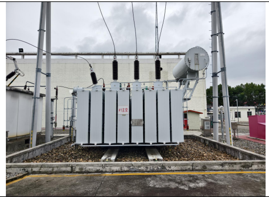
现有 1 号主变 (50MVA)
